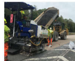
The UK's first carbon neutral pavement scheme used cold recycled asphalt mixed SuperLow asphalt, produced off site, to make a carbon neutral paving surface
